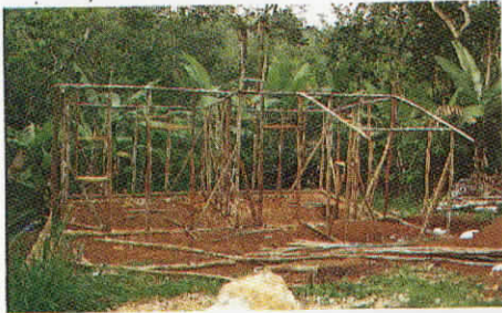
Framework for a concrete nog house. Note the wires strung between the posts for reinforcement.
