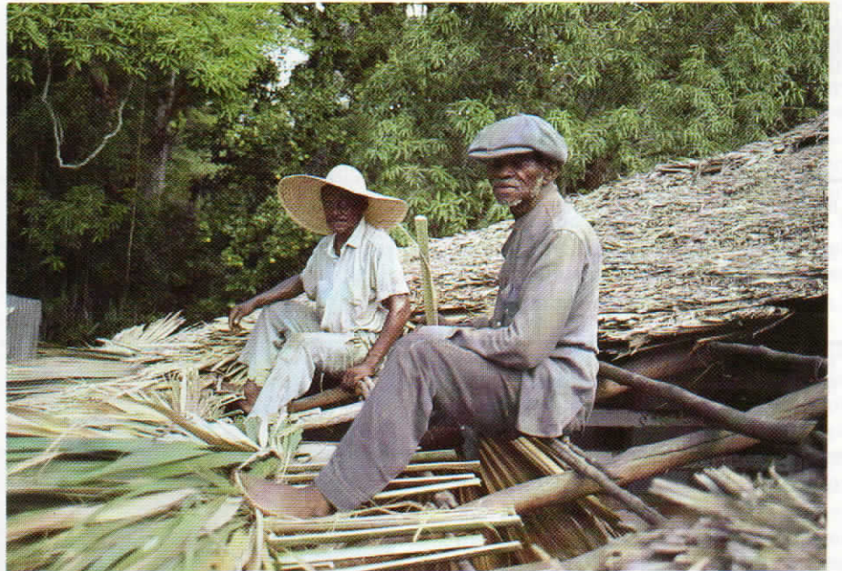
Two thatchers at work on a roof in St Elizabeth. Most of the craftsmen are now in their sixties and seventies; few young people are learning the skills.
