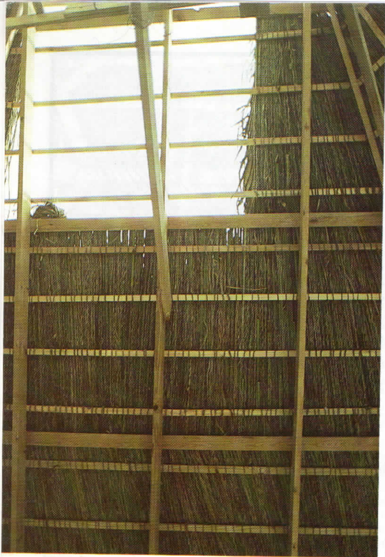
Underside of a roof thatched with Long Thatch tied on with wiss.
