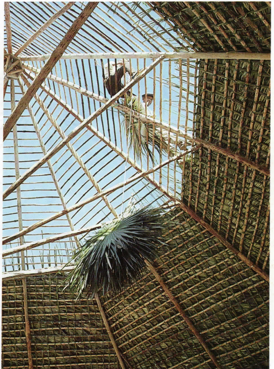
Thatchers at work on roof. Note thatch being hauled up by a rope.
